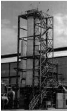
An ammonia converter 23 meters high installed at the Aonla plant in India by Haldor Topsøe. From Enriching the Earth .
